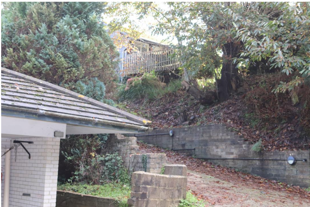
Photo 4.2: existing ramp and retaining walls fall partly within the application area and partly outside - the design proposals in this part of the site are unresolved and do not overcome the complex level changes
